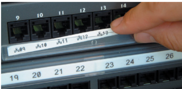
Punch block & patch panel labels
